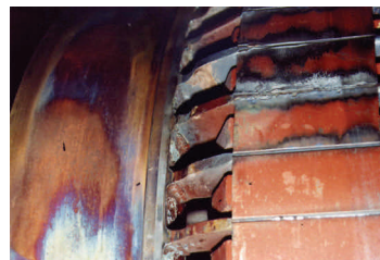
Rotor core damage due to broken bars
