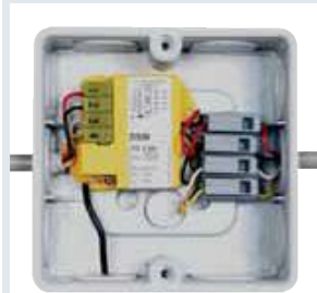
DSM installed in a surface-mounted distribution board
