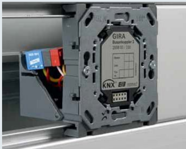
Protection of a KNX bus coupling unit by means of a BUSector surge arrester mounted on a bus terminal in the mounting area of a cable duct.
