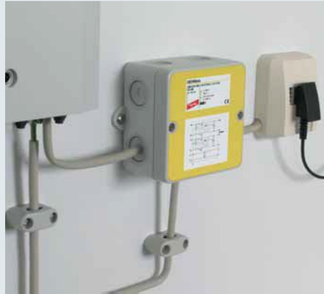
DEHNbox used for a telecommunication connection (example: U k0 interface)
