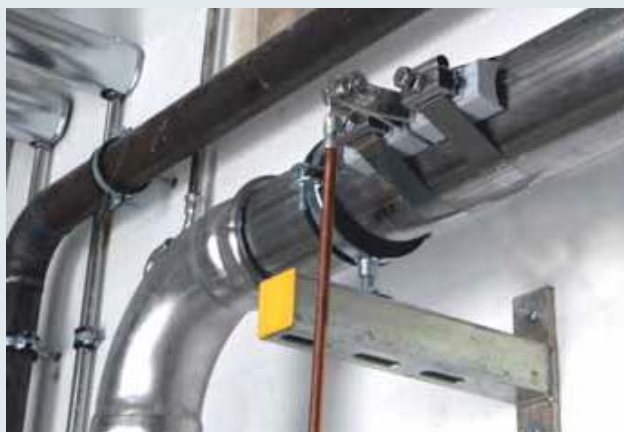
Applied at a StSt pipe
